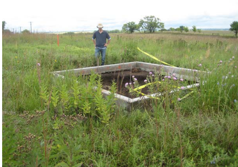
An idealized example of minimal-disturbance-footprint construction; small foundation within healthy old prairie.
